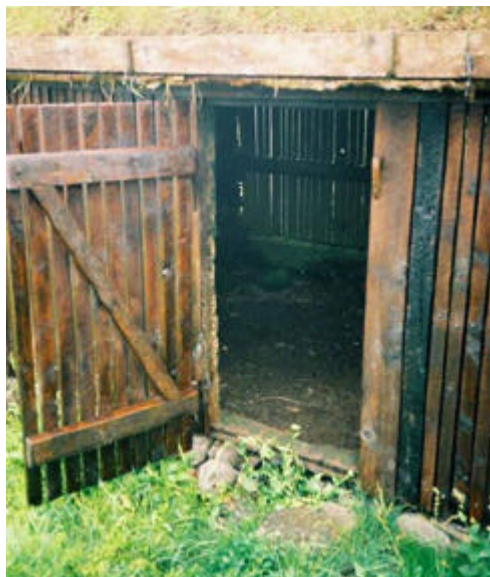
Fig. 4. Koltur's old buildings do not meet modern safety and access standards.
